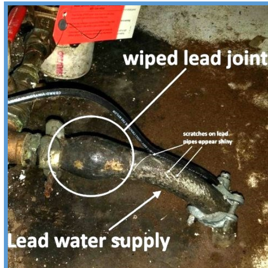
Lead service line right before the water meter
