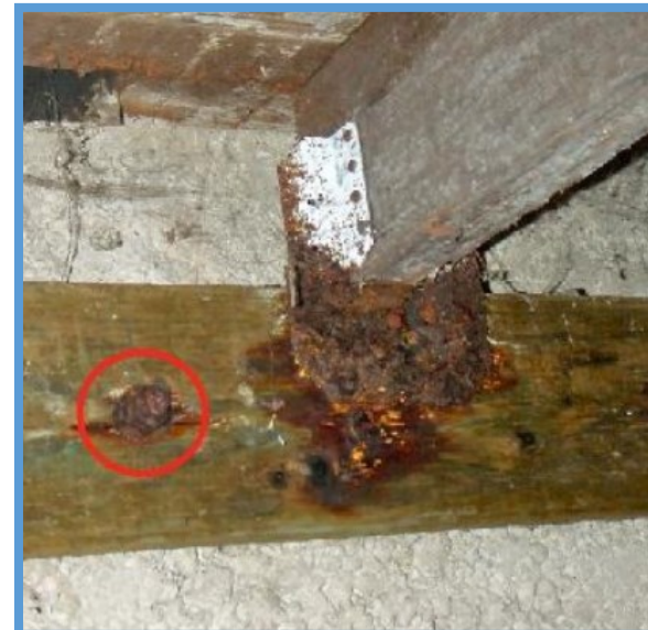
Look for rusted joist hanger and nails. The dissimilar metals iron in the steel connectors and copper in the lumber creates a galvanic reaction which causes corrosion
